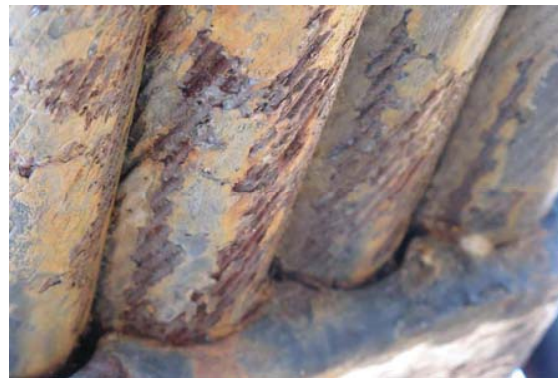
Figure 4. Detail of corroded cables.
